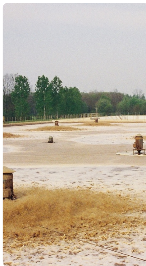
Airtec LFL aerators installed in an aerated lagoon
