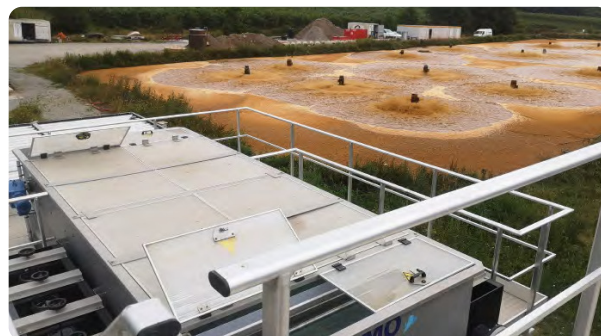
Gamtec unit on a high-flow industrial site
