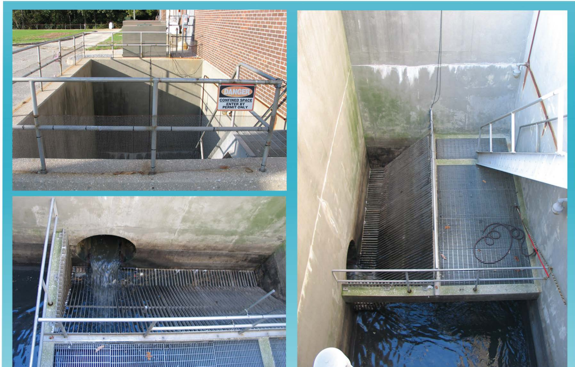
LTMUA Lift Station before Screentec.
